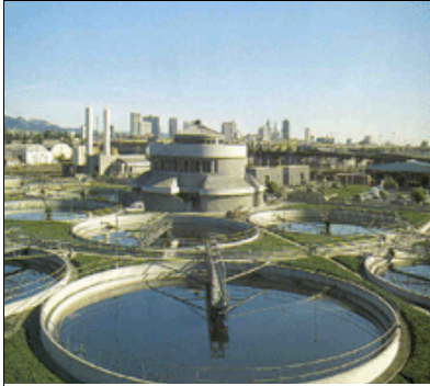
Clarifier at the EBMUD Wastewater Treatment Plant in Oakland
